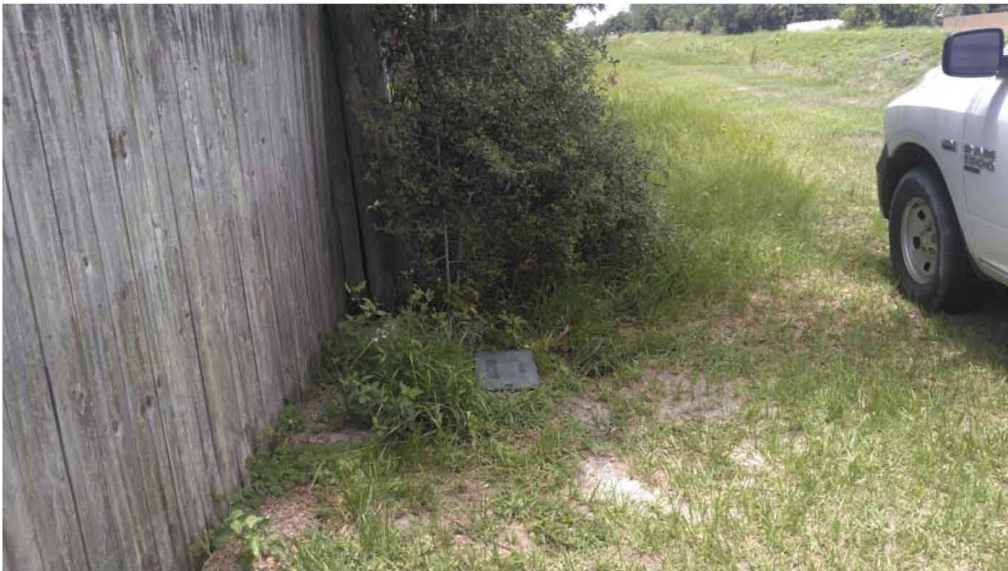
Handhole and pole at western terminus
