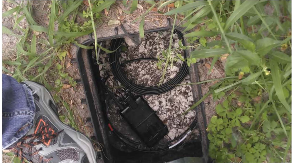
Handhole terminus at pole
