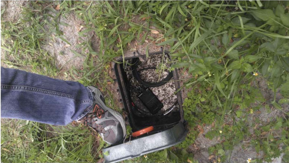
Handhole terminus at pole
