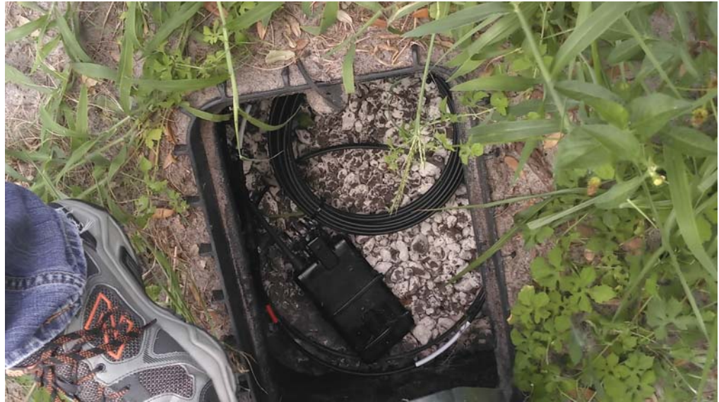
Handhole terminus at pole
