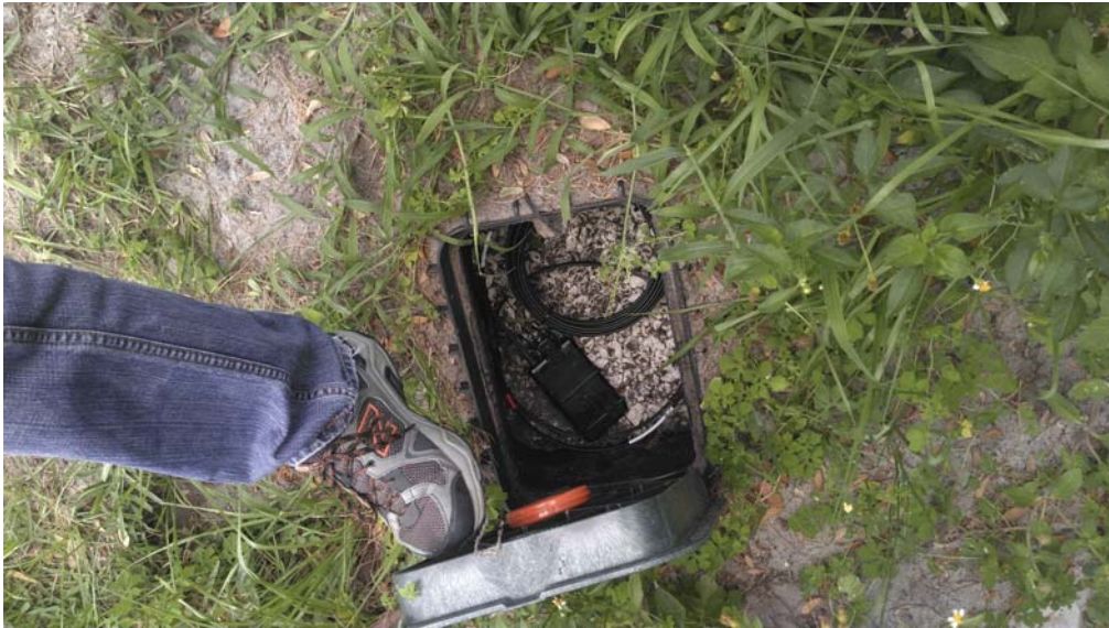
Handhole terminus at pole
