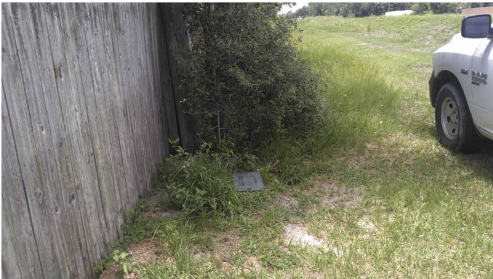
Handhole and pole at western terminus
